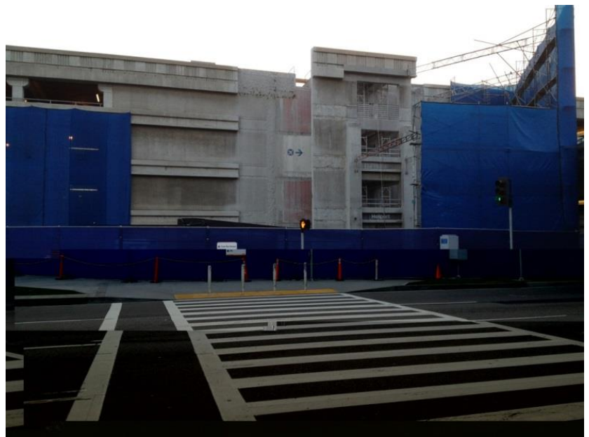
A blue construction barricade extending the length of Parking Structure 4 shows the impact the renovation is having on pedestrian walkways and access to the space.
