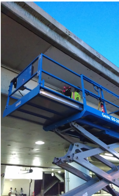
Workers use Ground Penetrating Radar Equipment to locate steel embedded in the concrete bridge structure of LAX's second level roadway.
